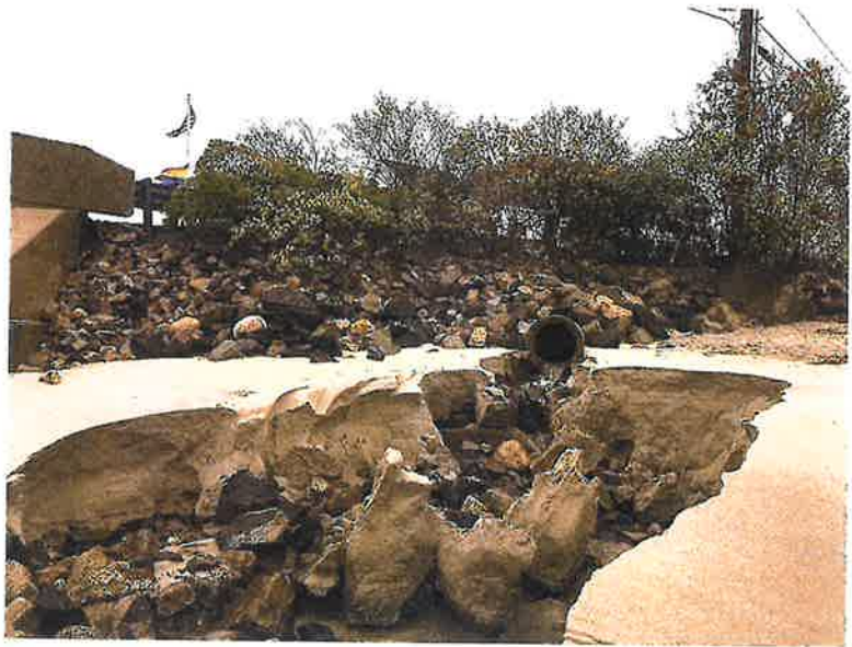
Outflow from OG-Pipe caused significant erosion during the Sep 30 th rain event.
